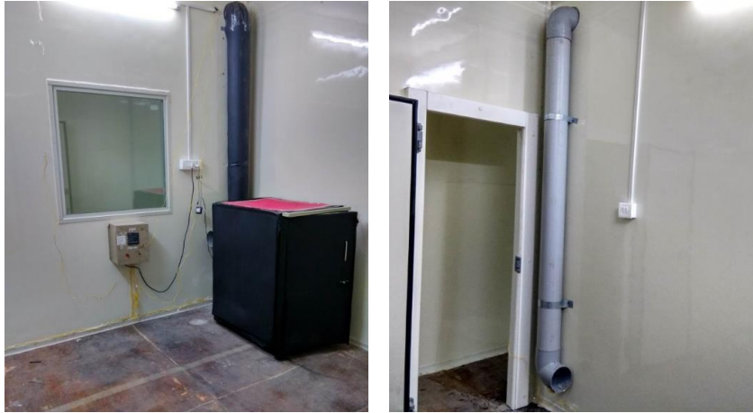
Figure 4: (L) Inside view of the inner room with HX, fan, data logger, and ducting (R) Sucking inlet of the room air
